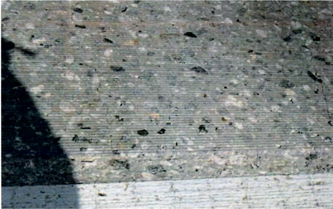
Figure A6-7. Existing Portland cement concrete (PCC) before and after grinding Consideration of existing pavement
